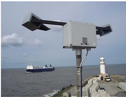
Navigation Lighting and Fog Horn Control
