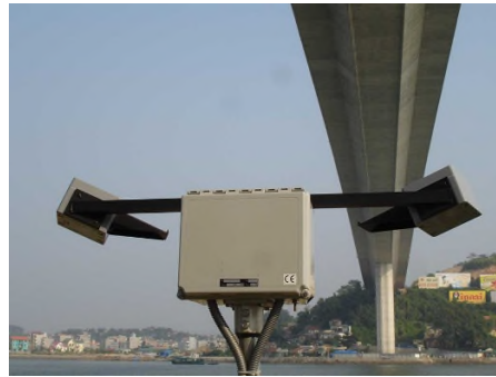
Bridge Visibility & Fog Warning Light Control
