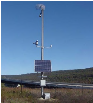
Road Weather Information Systems & Fog Warning Light Control
