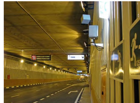
Tunnel Visibility Monitoring
